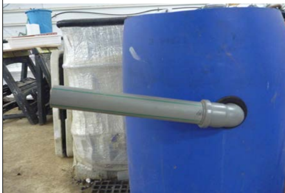
FIGURE 9.13 Overflow pipe on a biofilter
