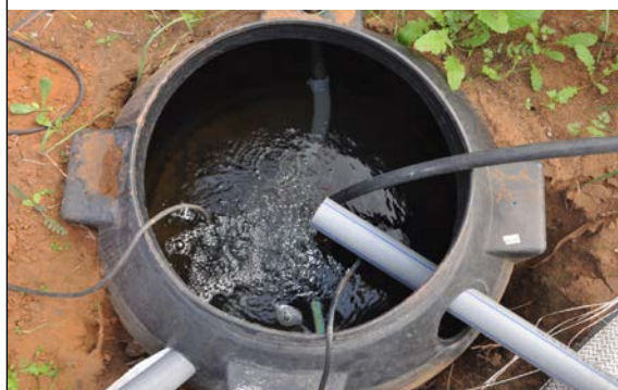
FIGURE 4.47 Sump tank buried in the ground to allow water collection by gravity
