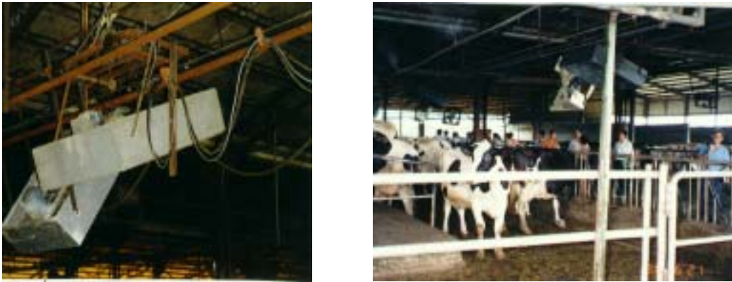
Figure 15. Movable fan installed with fogging on upper part of the dairy barn.
