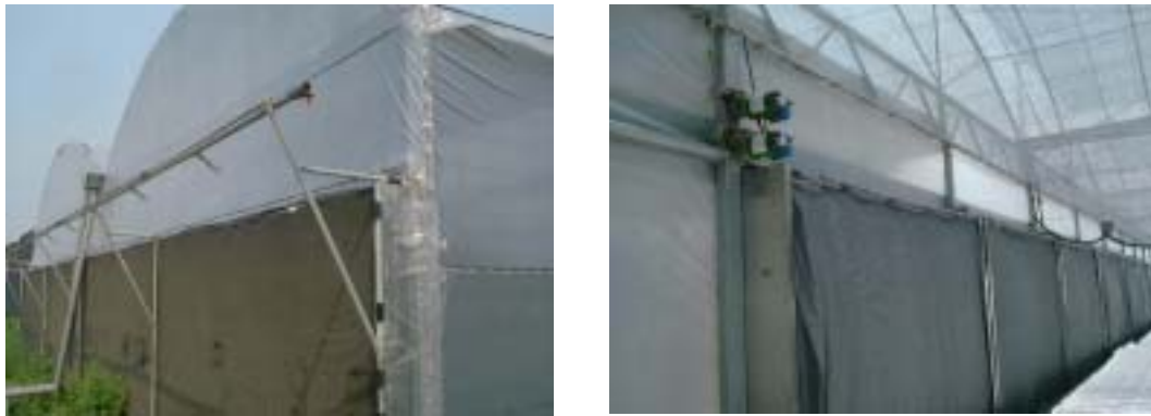
Figure 17a. Misting multi-layer net and fan system used in greenhouse (Fang and Lai, 2001).
