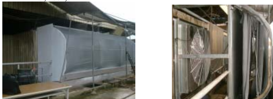
Figure 17b. Fogging multi-layer net and fan system used in dairy barn (Fang and Lai, 2001).
