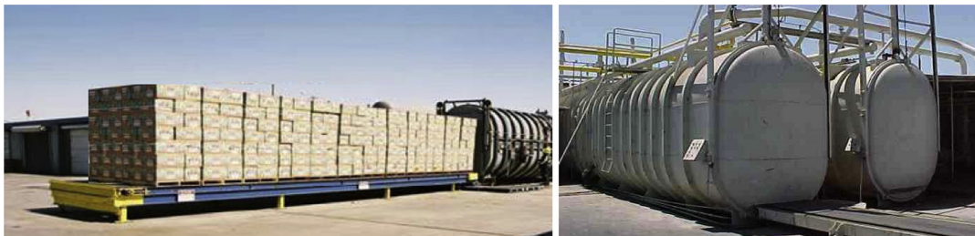
FIG. 6.19 Vacuum precooler during operation.
