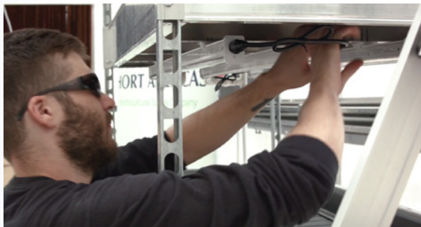
GE ARIZE LED Grow Lights Installation at Dallas Grown Greenhouse
